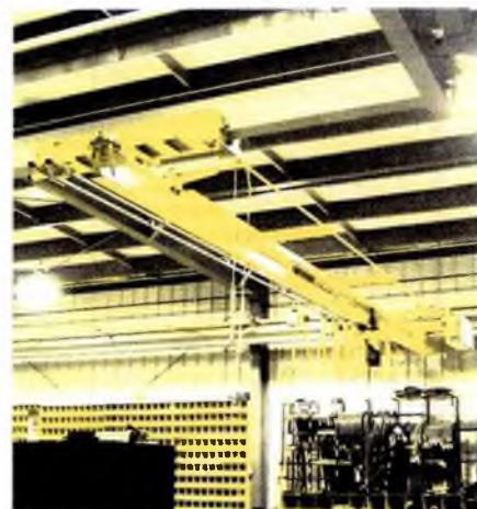
Figure 10: Overhead crane Source :
