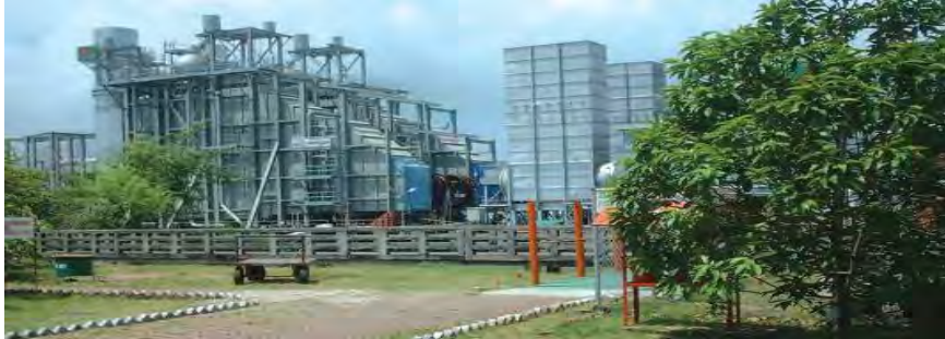
Power Generation Plant
