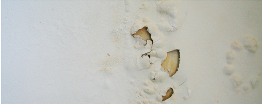
Figure 2.6.1: Dampness in wall. Source ( http://www.risingdamp.co.uk )
