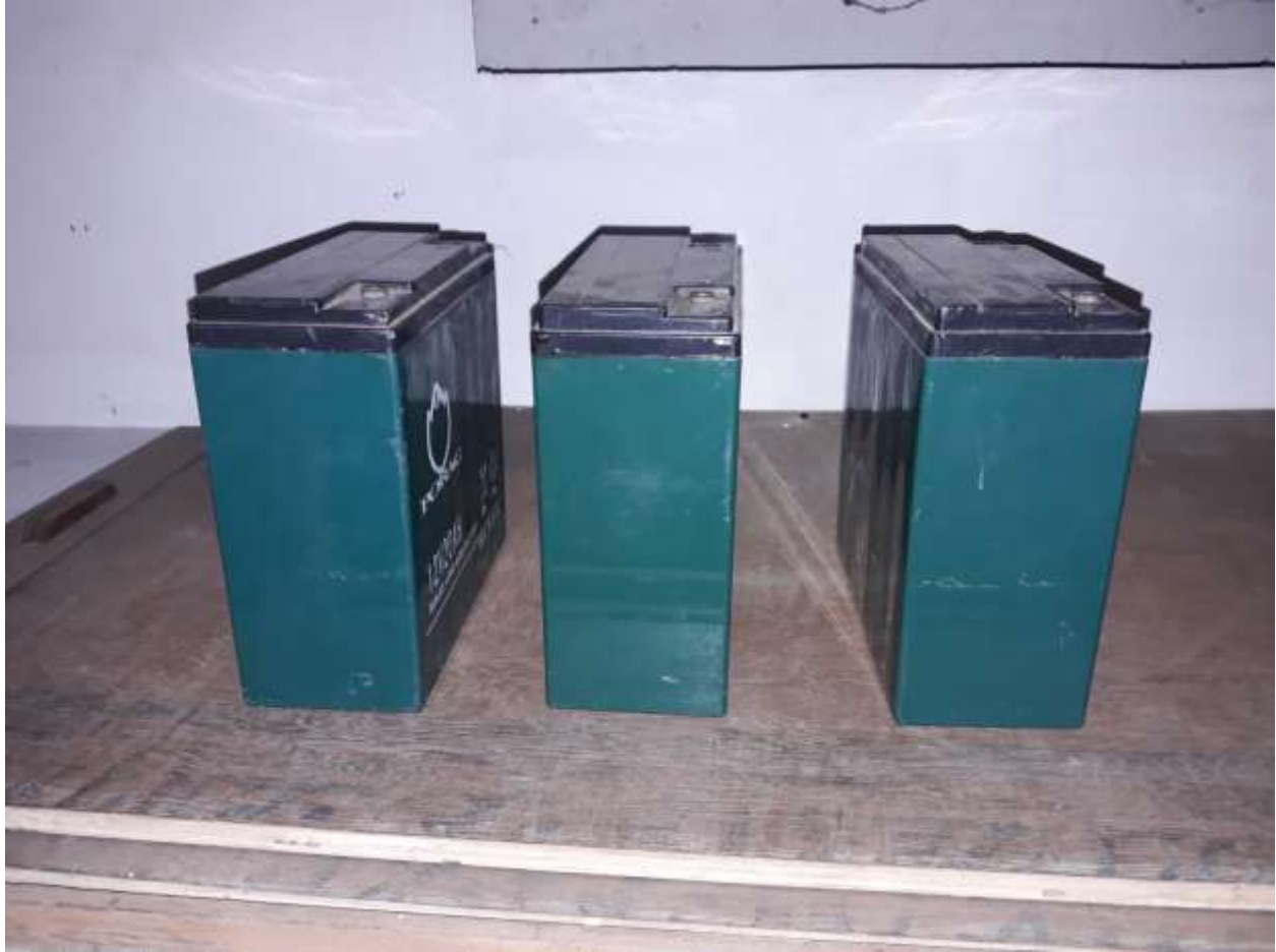
Fig 3.4: Batteries for solar heater
