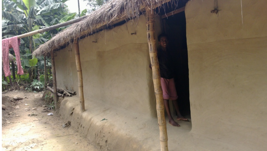
Picture 11: House made of mud wall and sun grass by tea laborer
