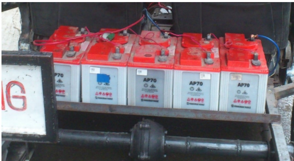
Batteries placed in the back of the car
