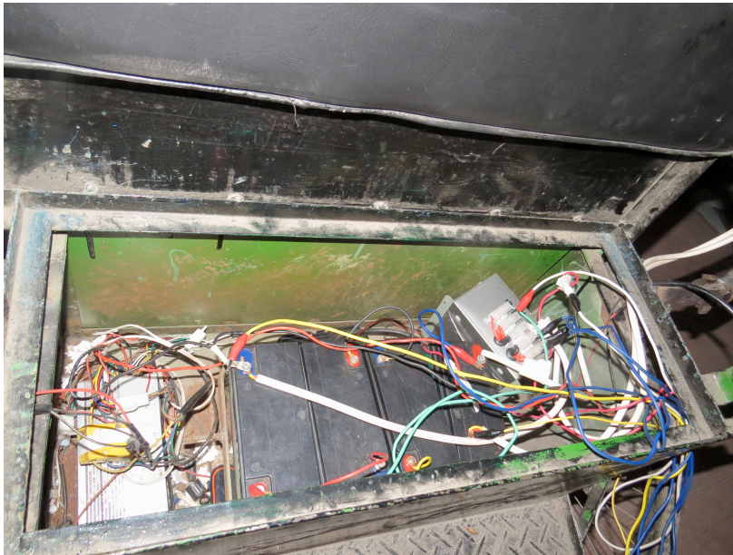
FIG. 3.3 4, 12V BATTERIES IN SERIES
