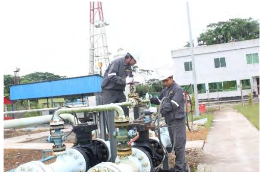
Gas Process Plant Maintenance
