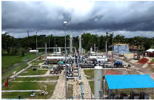
Shahbazpur Glycol Type Gas Process Plant
