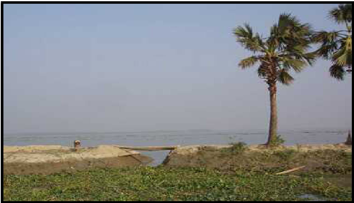
Figure 2.3: Broken Embankment before Sidr in kalapara Source: Shibayama T. 2008
