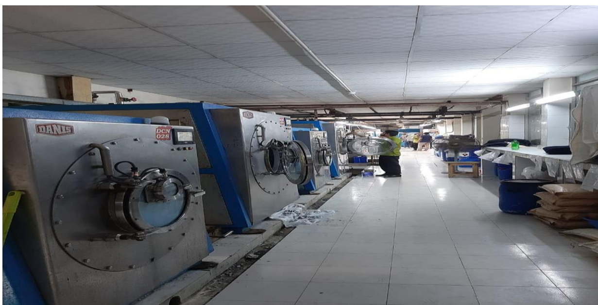
Fig no-11: Washing plant (Photo by Atiqur in August 1,2022)
