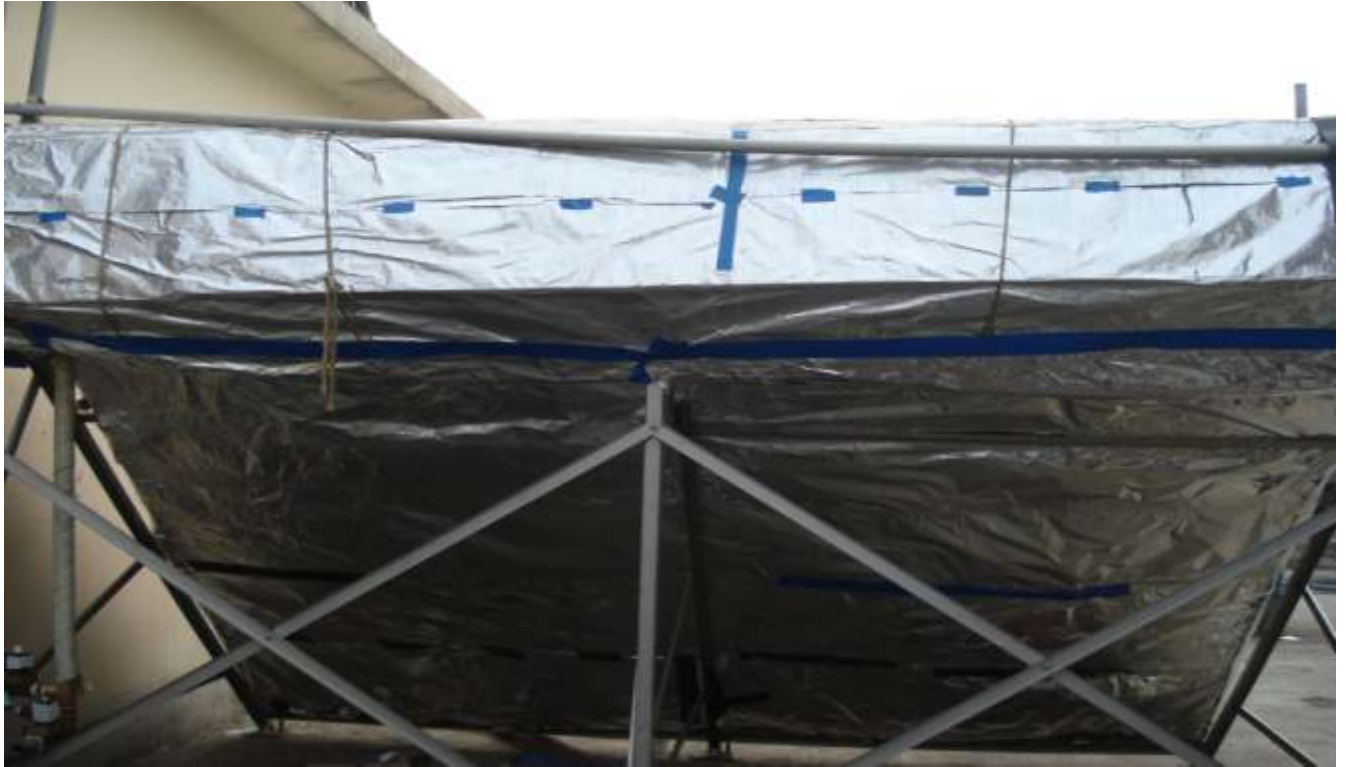
Fig 16: Back view of the storage tank
