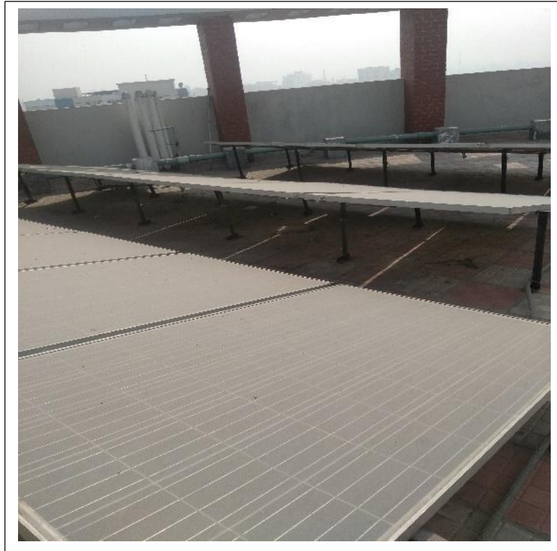
Figure 2.19: Solar Panel from first apartment of Faridabad (side-view)
