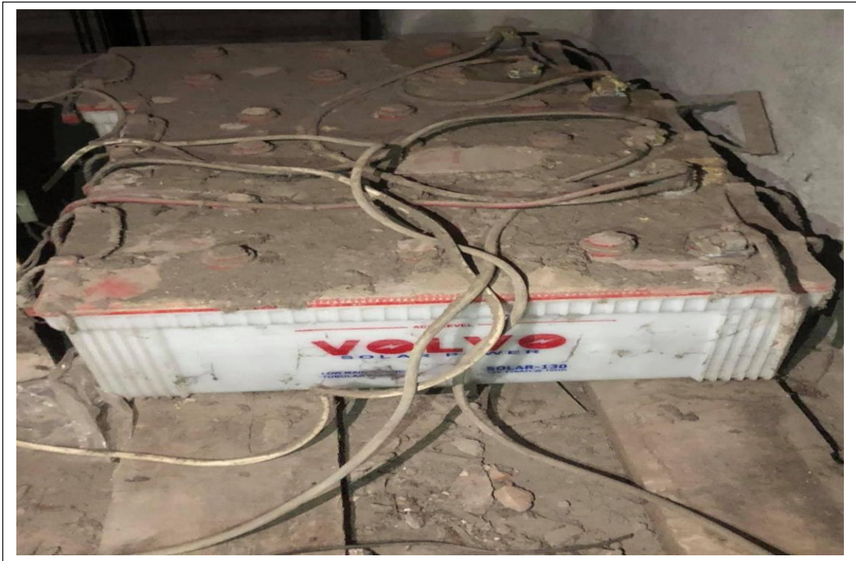
Figure 2.5: Battery from apartment of Mohammadpur
