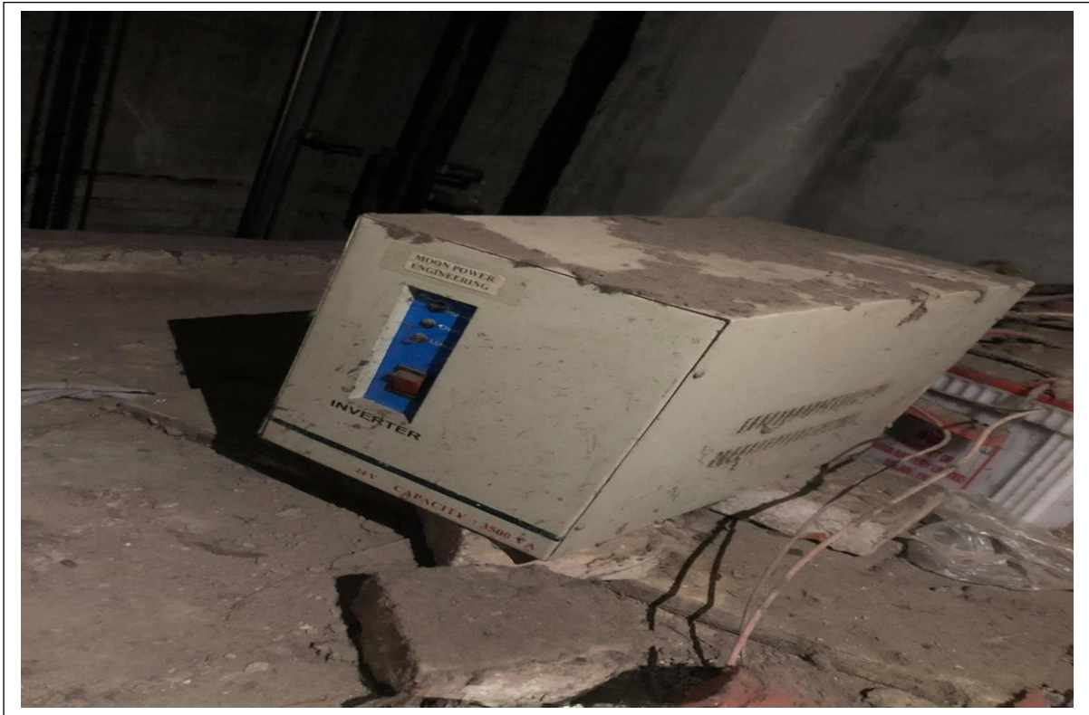
Figure 2.4: Inverter from apartment of Mohammadpur
