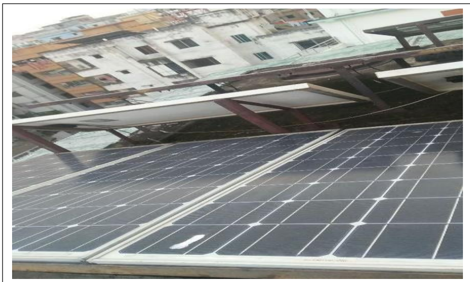
Figure 2.9: Solar Panels from apartment of Shyamoli (Front view)
