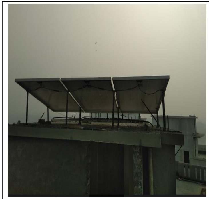
Figure 2.26: Solar Panel from second apartment of Faridabad (lower-view)
