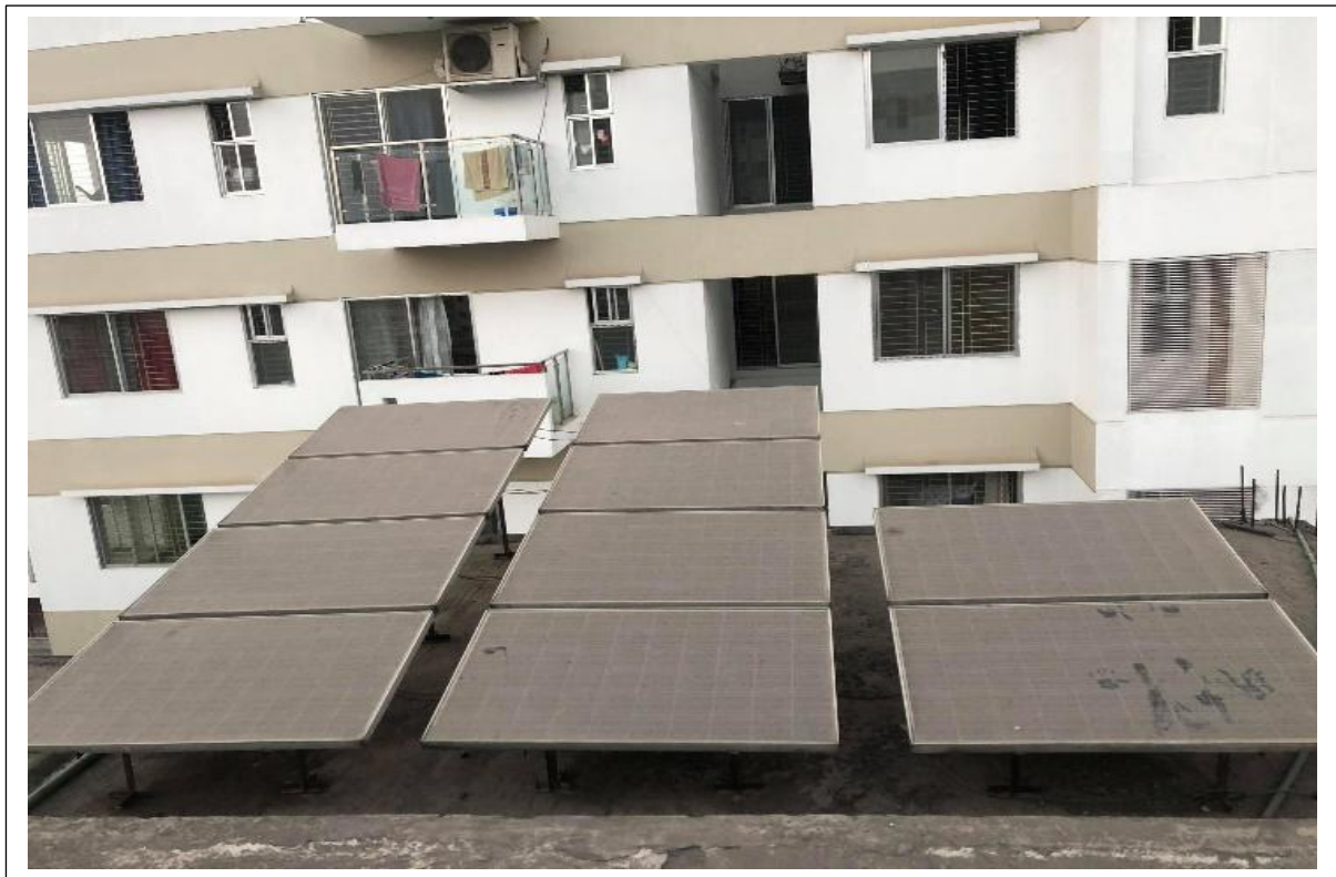
Figure 2.1: Solar Panels from apartment of Mohammadpur
