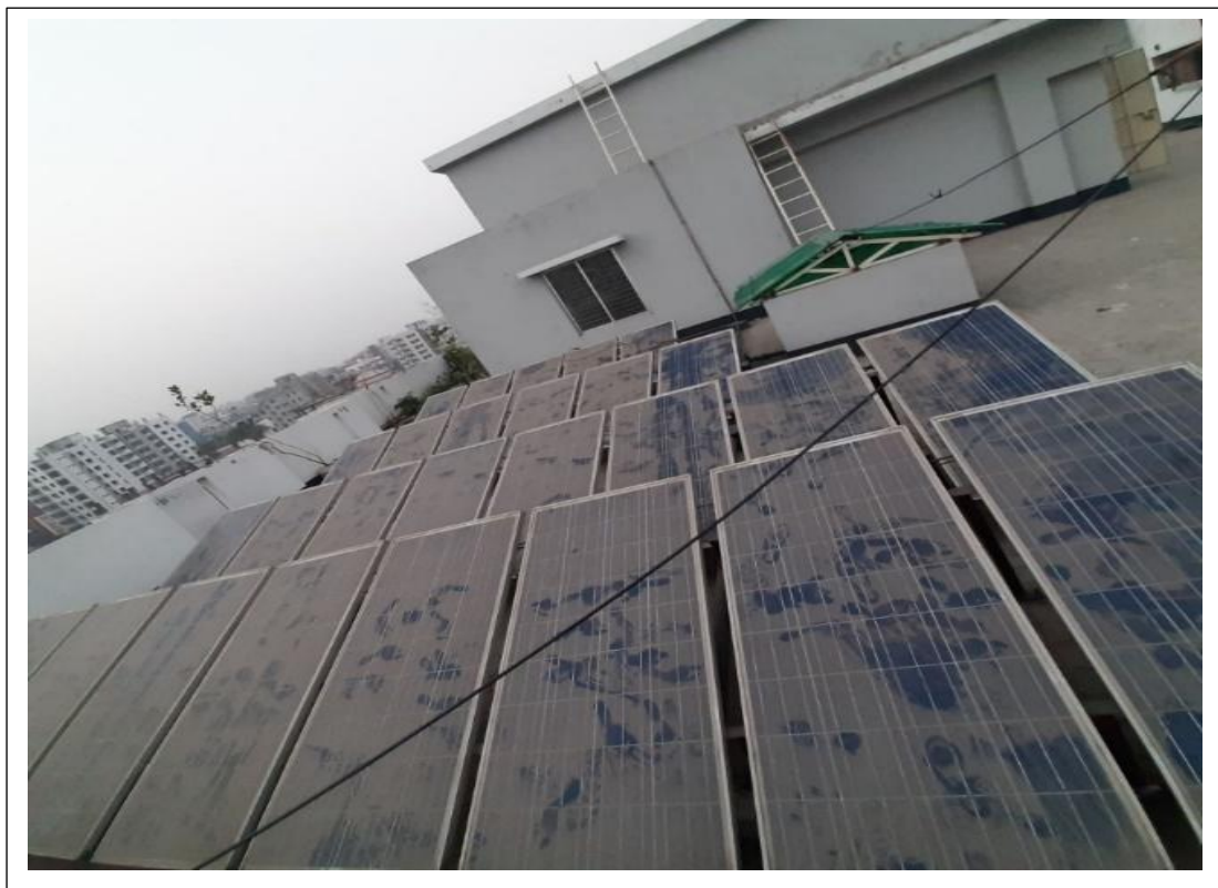
Figure 2.12: Solar Panels from apartment of Agargaon
