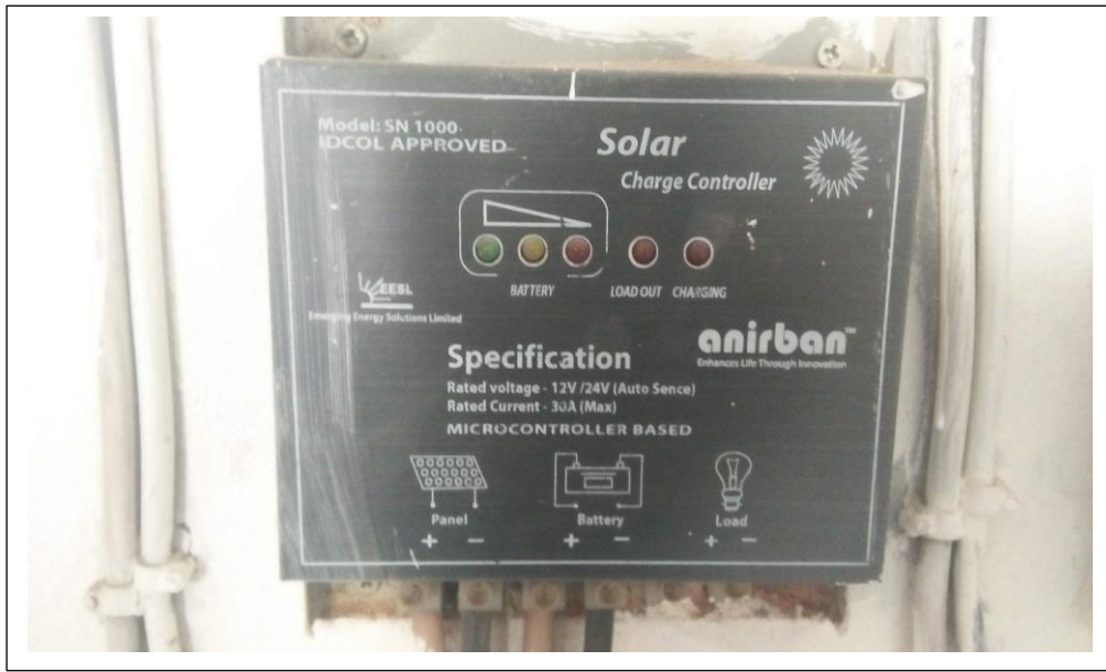
Figure 2.11: Solar Charge controller from apartment of Shyamoli
