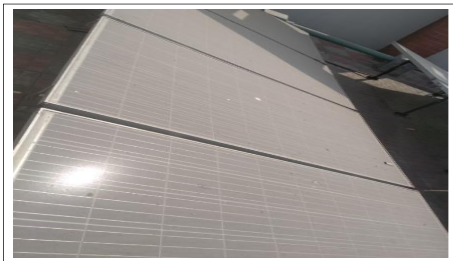
Figure 2.18: Solar Panel from first apartment of Faridabad (upper view)
