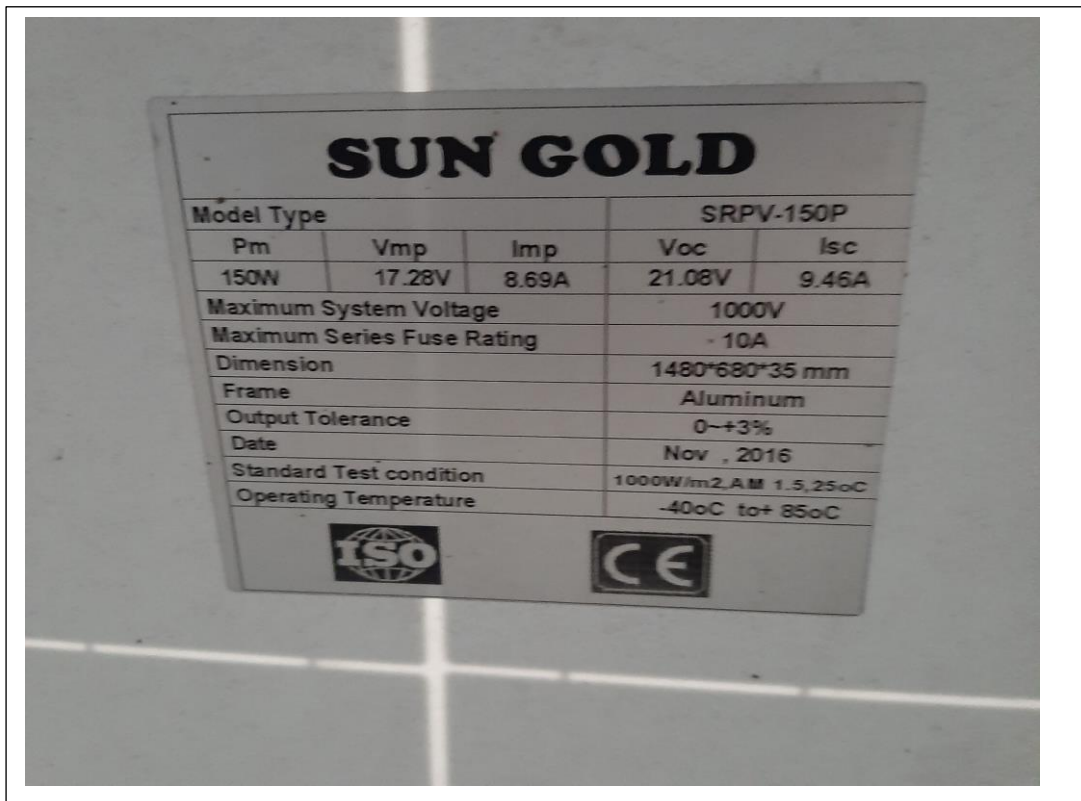
Figure 2.13: Solar Panels ratings from apartment of Agargaon
