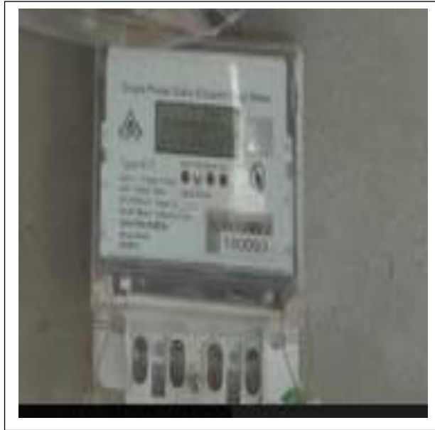
Figure 2.31: Meter from 2 nd apartment of Faridabad
