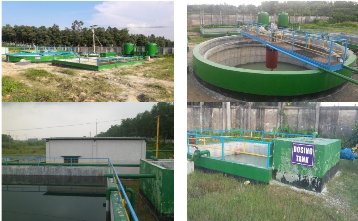
Sewage Treatment Plant
