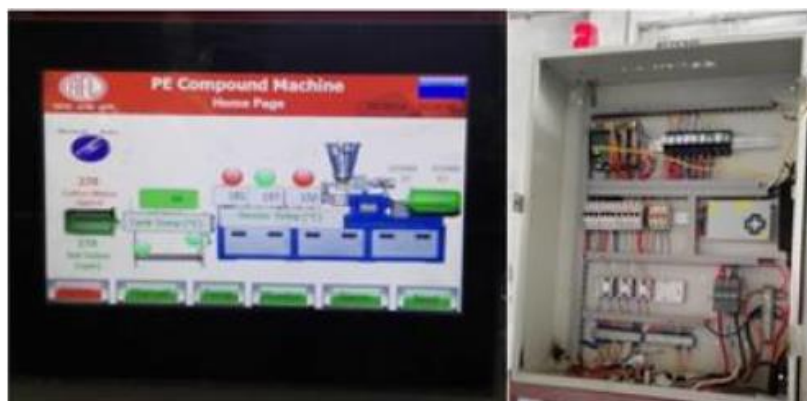
Figure-4.2(a): Automation in PE Compound machine of kitchen shelf plastic paint resin with PLC & HMI
