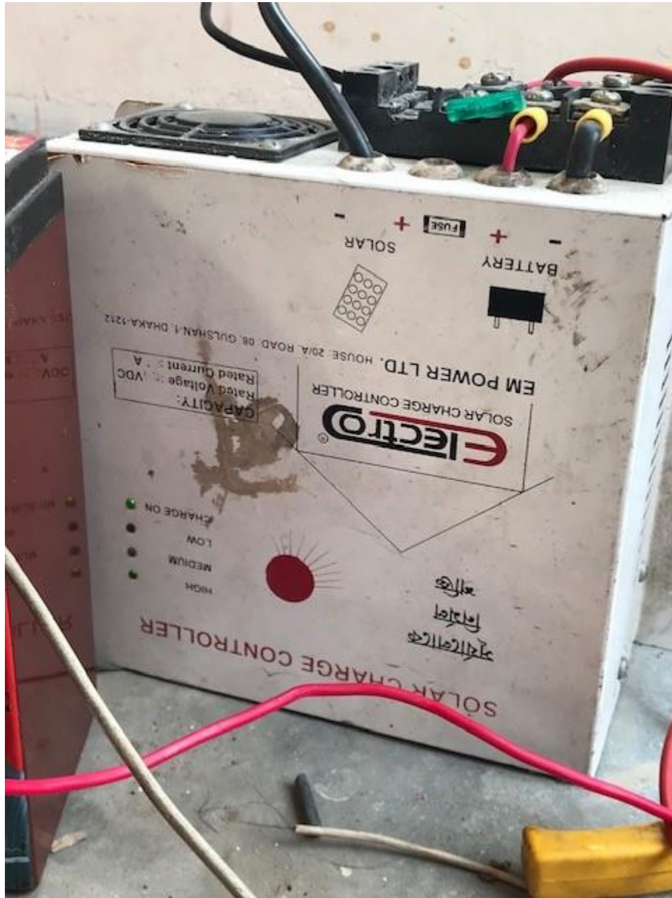
Fig 2.16: Electro Charge Controller
