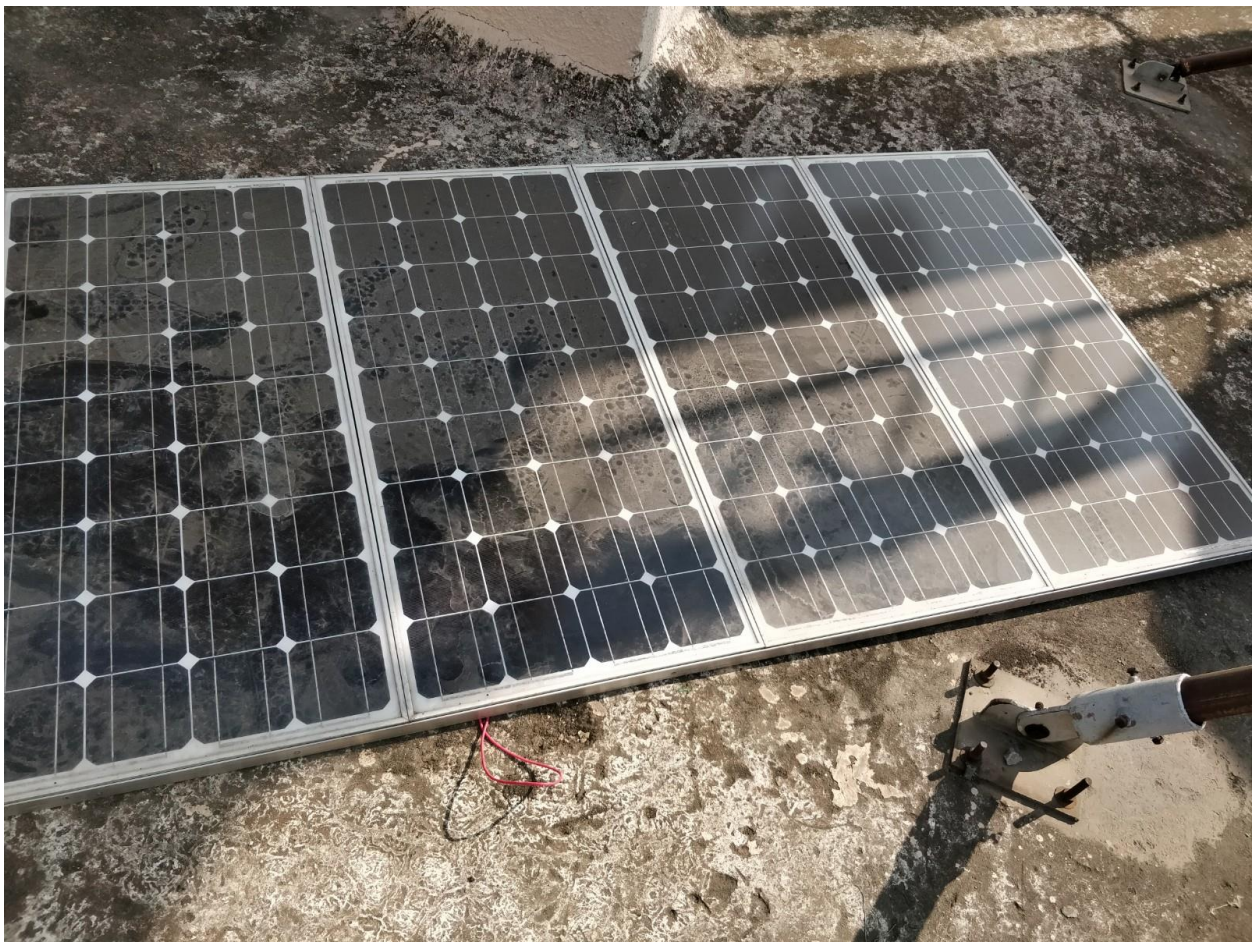
. Fig 5.1: The Solar Panels used for the Solar Charging Station
