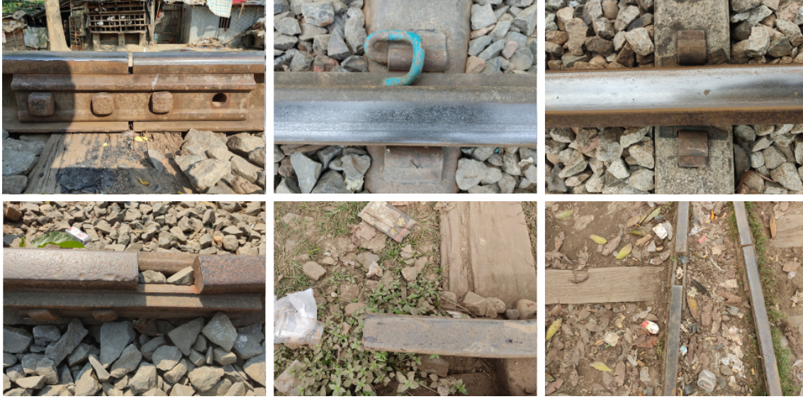
Figure 4.2: Samples of faults on railway tracks
