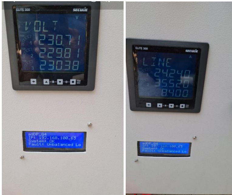
Figure 5.30: Transformer real value in the device.
