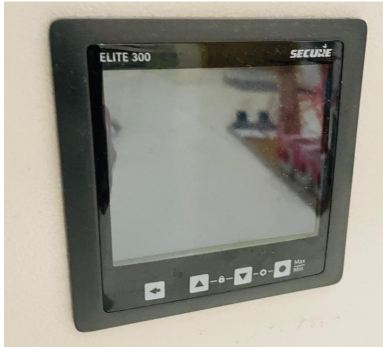
Figure 5.2: Multifunction Panel Meter
