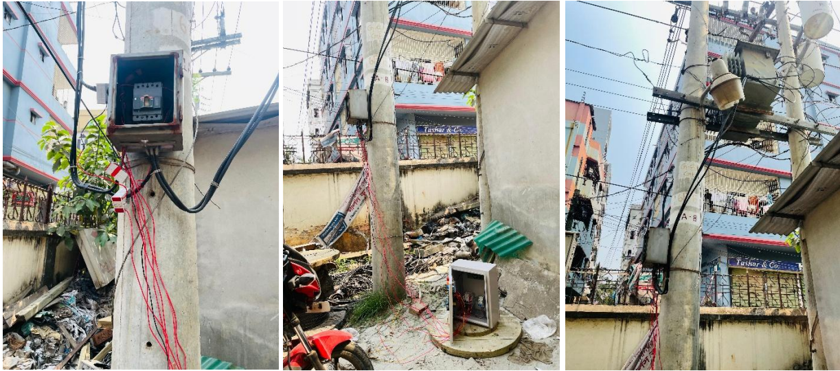
Figure 5.28: From Left, CT connection in the MCB Load side, Full system connected in the Transformer, and 100KVA Transformer at BREB Campus (Dhaka PBS-03)
