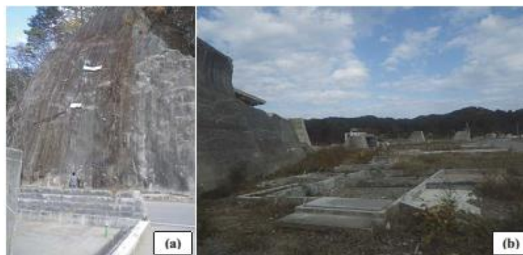
Figure 56 (a) Height records of historical tsunamis in 1896 & 1933 (b) destroyed sea walls in 2011 (Source: Journal NDS, 2012)
