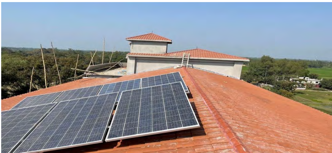
Figure 13 : Solar energy using in roof top in newly constructed educational building
