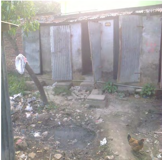
Pic 3: Filthy toilets
