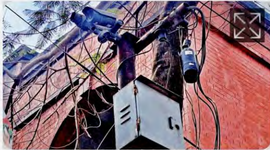
An inoperative CCTV camera in Barishal city. Photo: Titu Das
