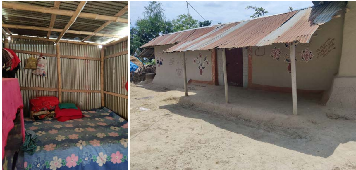
[Image 1 & 2: Indoor of a house: tin-made wall and ceiling with no ventilation; Outdoor of a house: mud wall and floor with tin roof]
