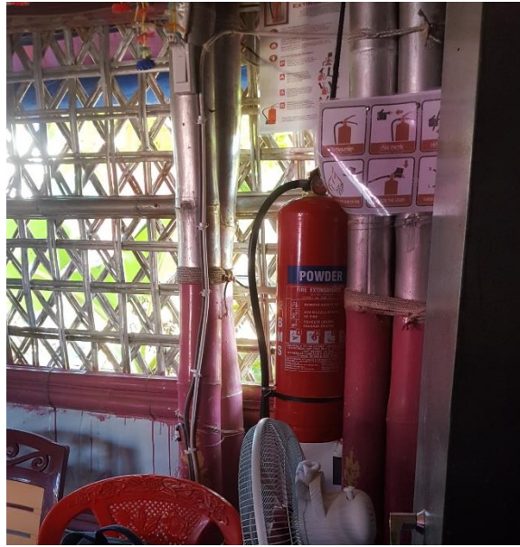
Figure 23: Image of a fire extinguisher at CFS. Source: Field survey by Author, 2020
