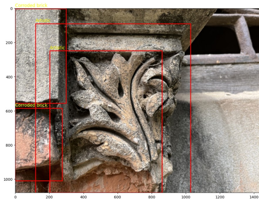
Figure 5.2: Sample image of Corroded brick from the heritage dataset[18]
