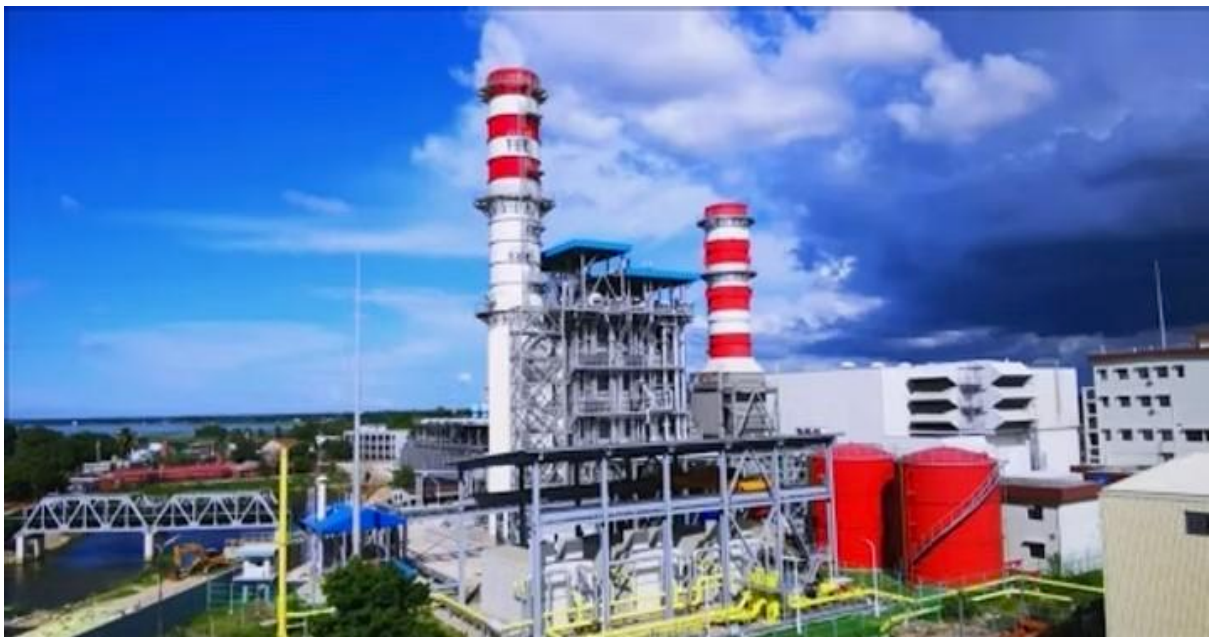
Fig. 4.8 400 MW CCPP (East) Plant
