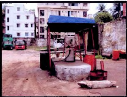
Fig 13: Existing Diesel Pump Source: Hoque, 2011
