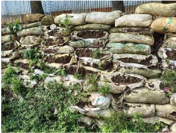
Fig-36: Damaged earth-filled sack protection wall
