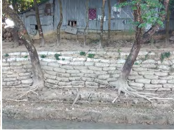
Fig-37: Earth-filled sack protection wall
