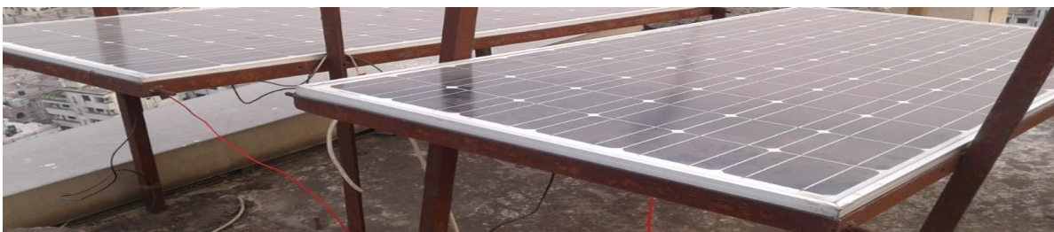
Fig 6.1: Solar panels being charged on the rooftop of BRAC University
