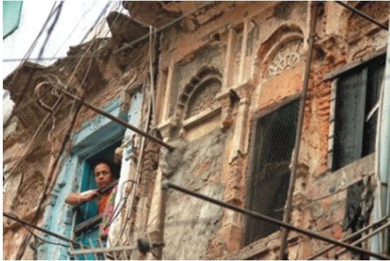
Figure 5: The poor condition of the heritage buildings Photograph: Iftekhar Ahmed
