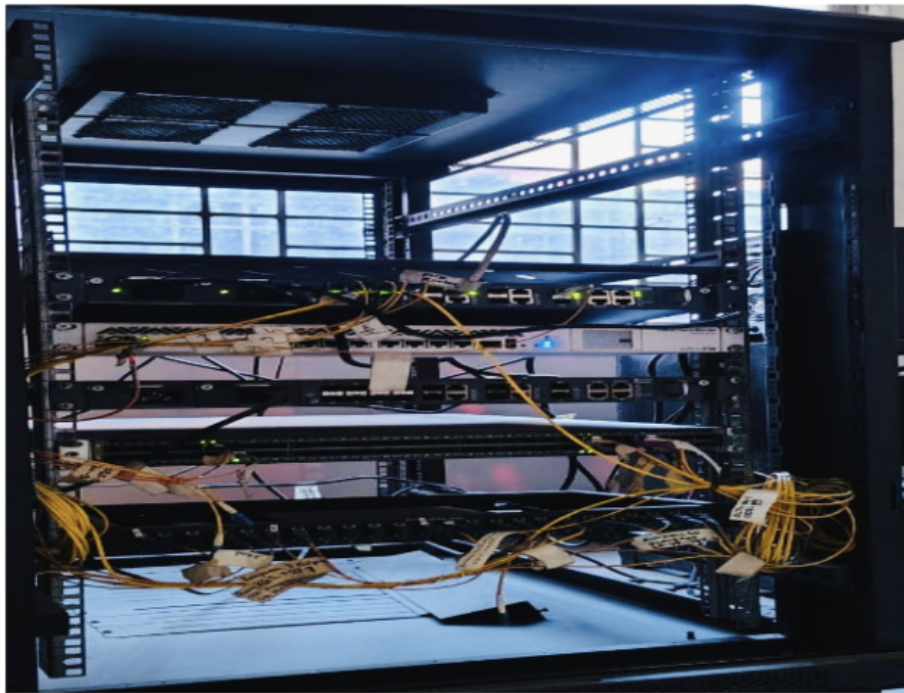
Figure 4.2: Optical Line Termination
