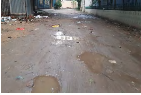
Figure 5.15: Pothole in Concrete Road
