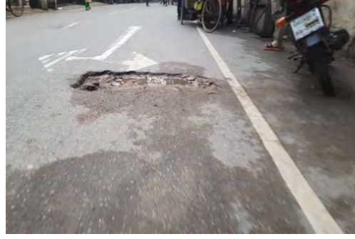
Figure 5.16: Pothole in Paved Road
