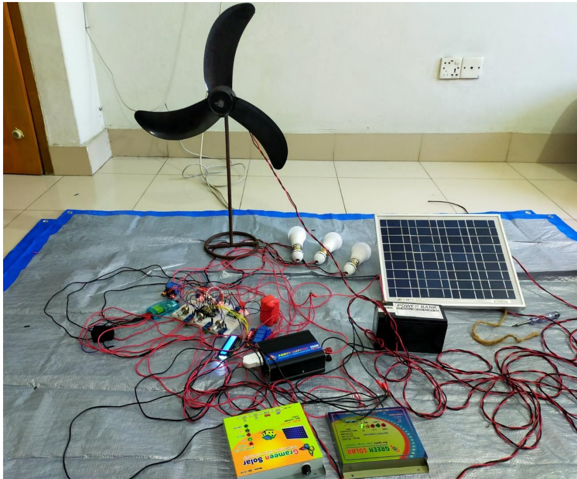
Figure 4.8: Complete Circuit Setup View
