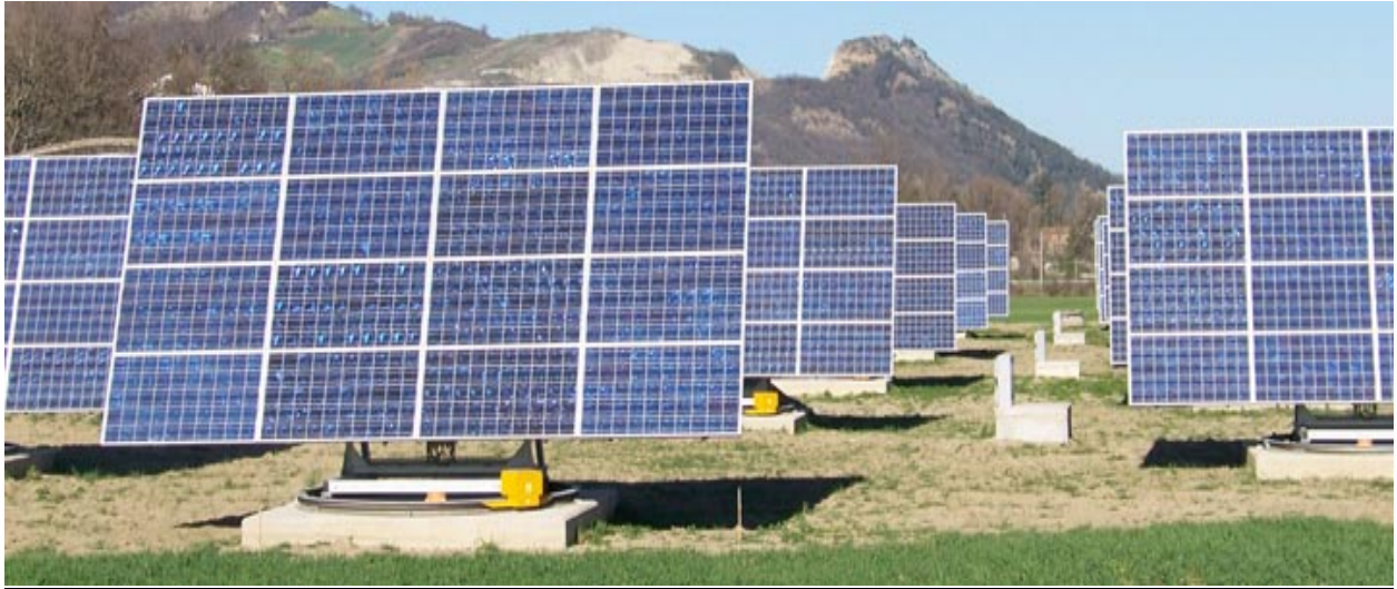
Figure 1: Photovoltaic (PV) Solar system
