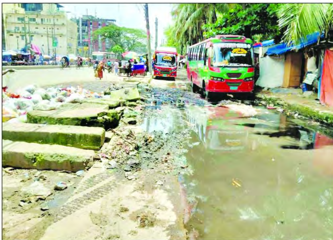
The busy main road beside the Dhaka South City Corporation office has been left in tatters with potholes and dumping of garbages and concrete slabs posing the risk of serious accidents at anytime. The photo was taken from Gulistan area on Wednesday. ■ Photo: Moin Ahmed
