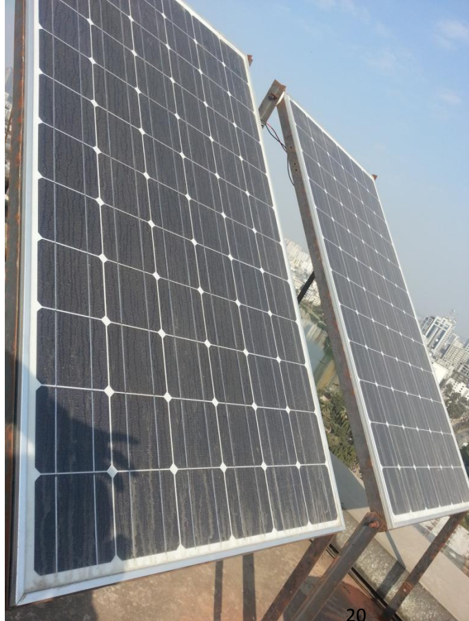
Fig 3.3: The Solar PV Panels
