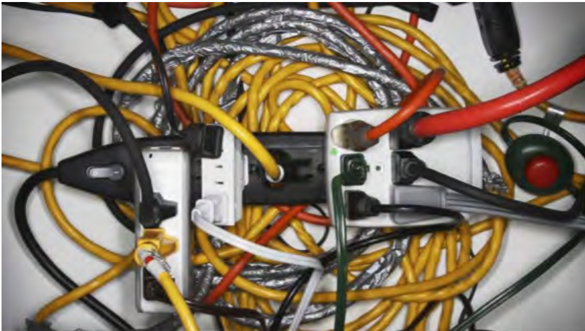
Fig. 1.2 Wired charging system [39]
