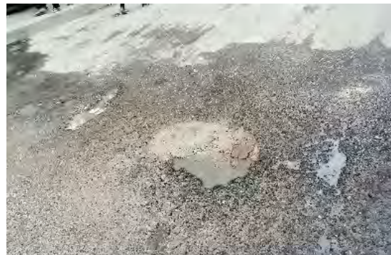
Figure 4.4 - Potholes in wet road
