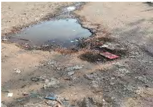
Figure 4.1- Potholes filled with sand or polyethene or any other disturbance.
