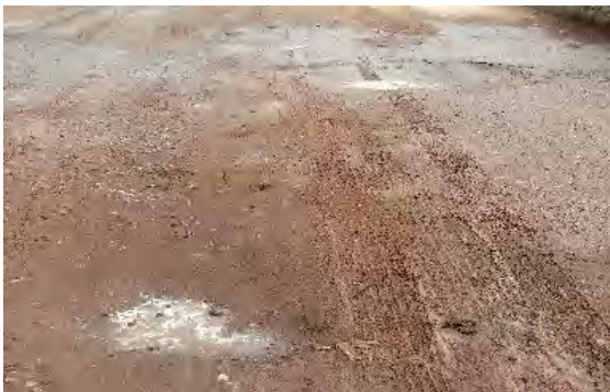
Figure 4.3 - Potholes in muddy or earth road
