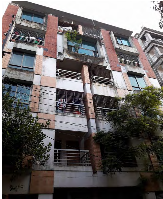
Fig: F. No maintenance of exterior facade a.c. outdoor unit
