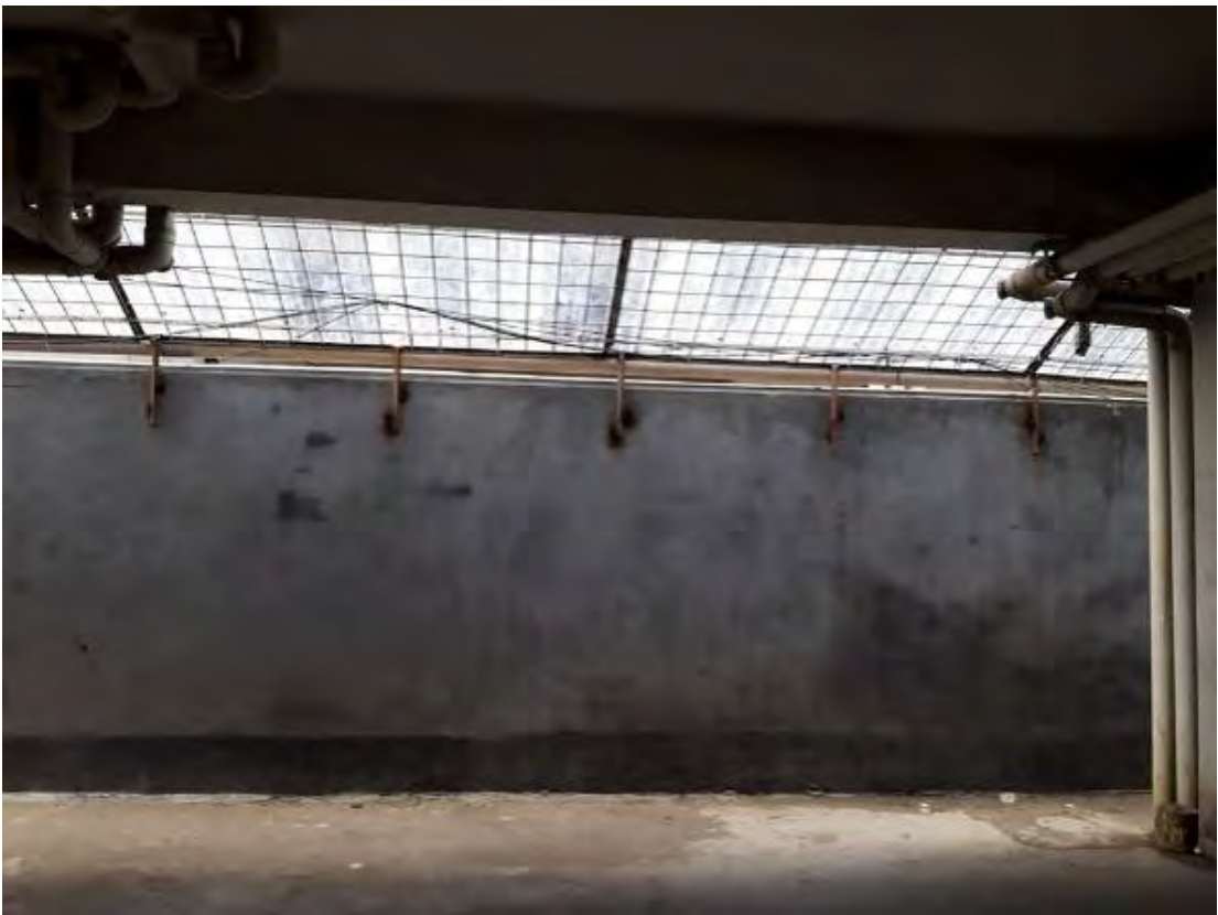
Fig: H. Violation of building code by covering the setback units for adjoining the two units.area with asbestos sheets.
