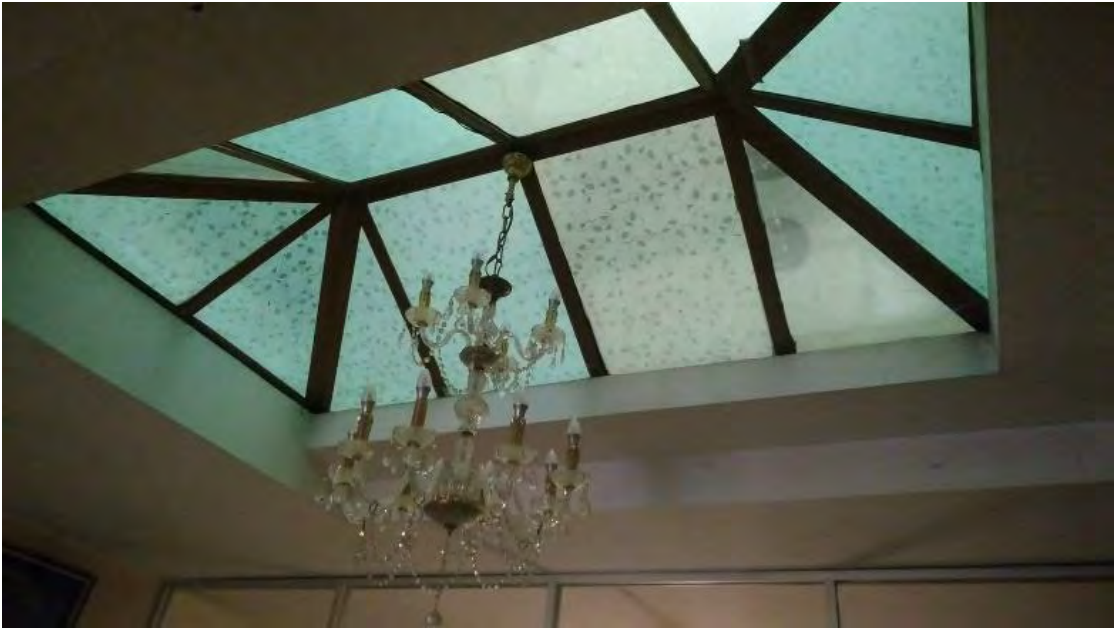
Fig: G. Violation of building code by covering up the void space between two
