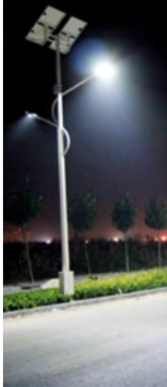
Figure 6.3: Decentralized Solar Street Lighting System
