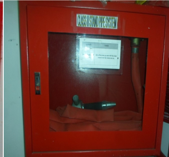
Fire Hose Reel
