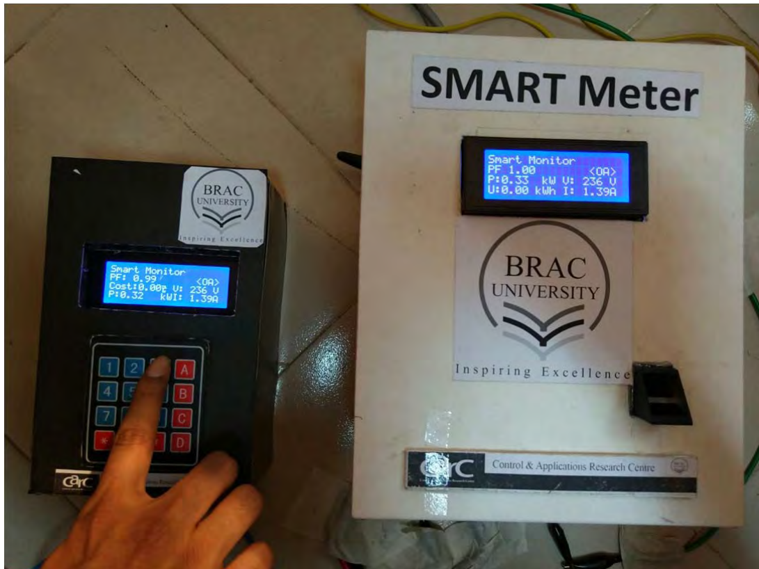
Figure 7.4: Getting Overall Electricity Consumption from Meter
