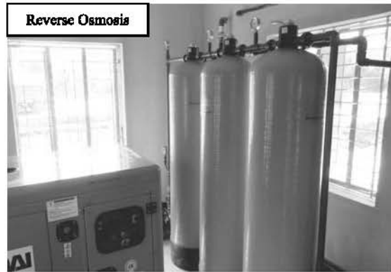
Fig 5: Examples of installed water technologies in different HiR areas by NGO Forum.
