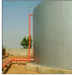
Fire water tank incl. fire water piping
