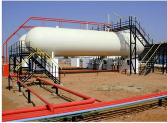
Above ground storage tank incl. fire water piping
