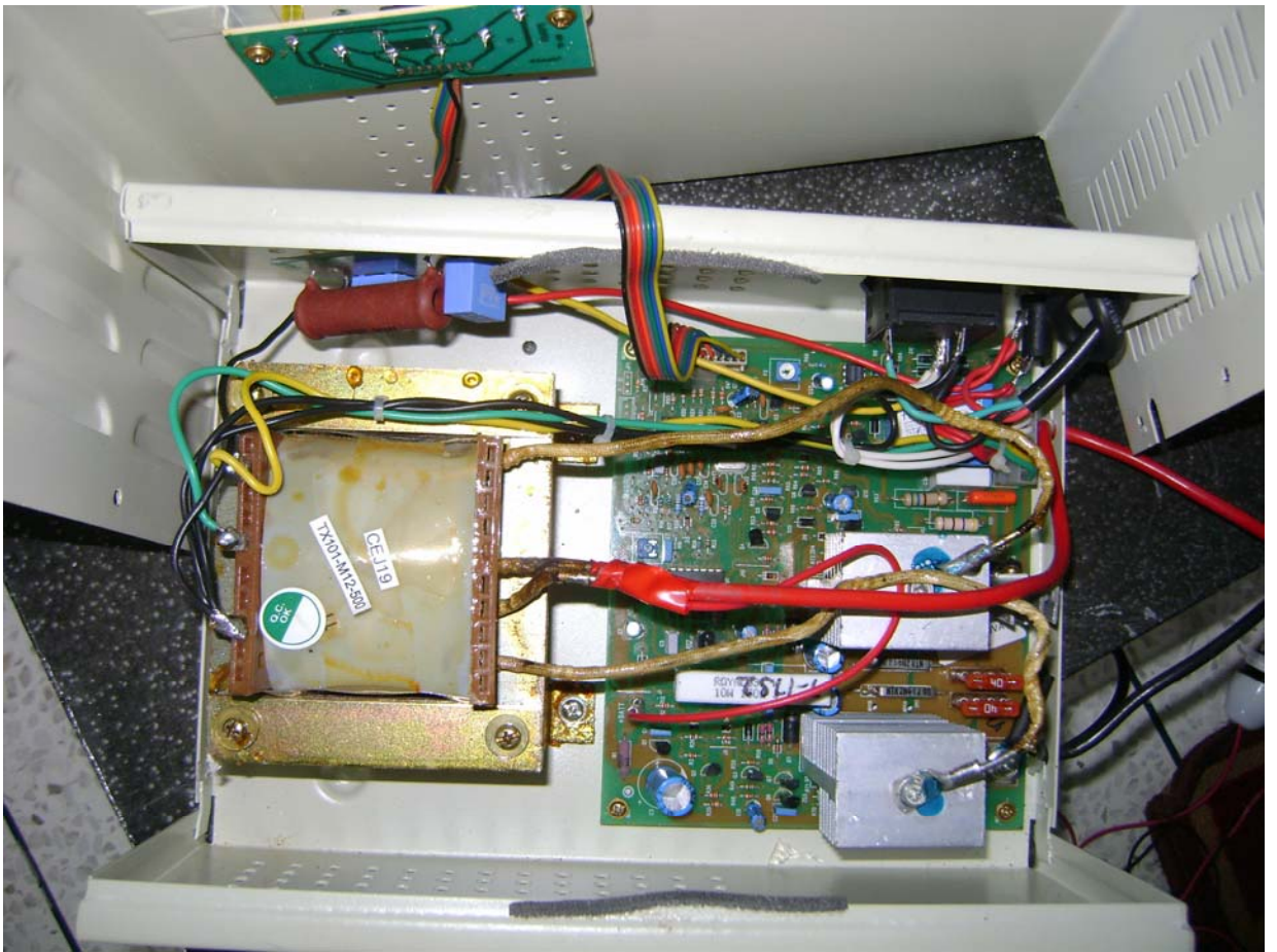
Internal Circuitry of IPS
