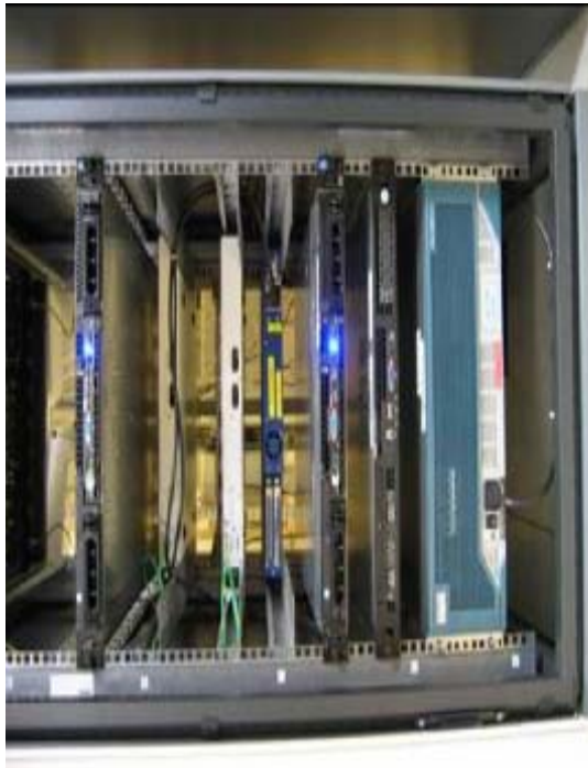
Figure 4.5: WiMAX Access Controller (WAC) cabinet
