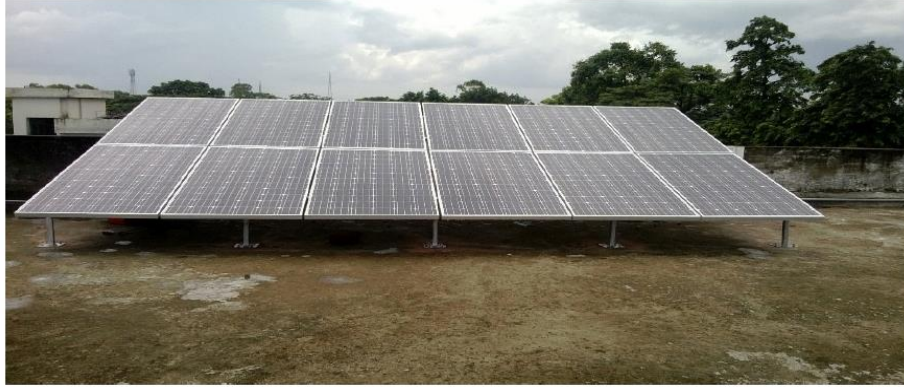
Figure 2.6: Solar AC System (Off Grid) installed at Mawna, Gazipur
