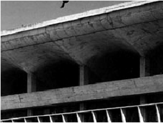
Figure 19 Double roof, High Court
