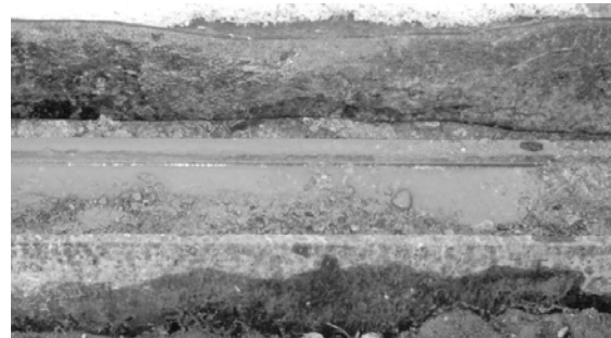
Figure 6: Microbial corrosion underneath train rails.
