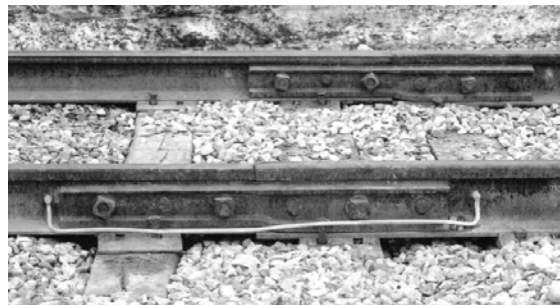
Figure 4: Crevice corrosion between train rails and metal connectors.
