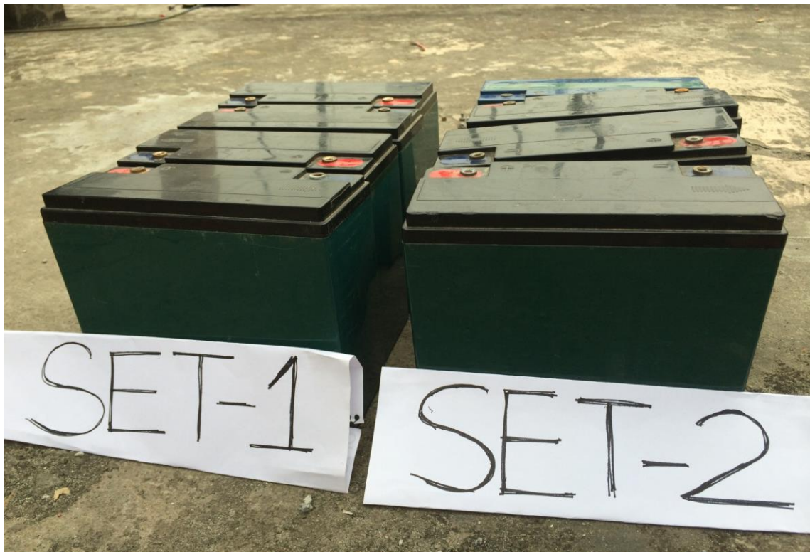
Figure 5.2: Two sets of 48 V batteries
