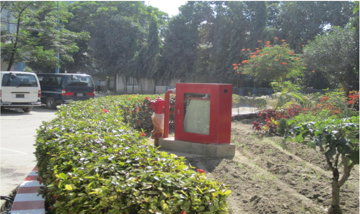
Figure 13-3: Fire Hydrants Point
